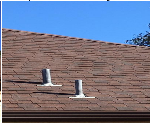
Rusted exposed nail heads need roofing cement.
