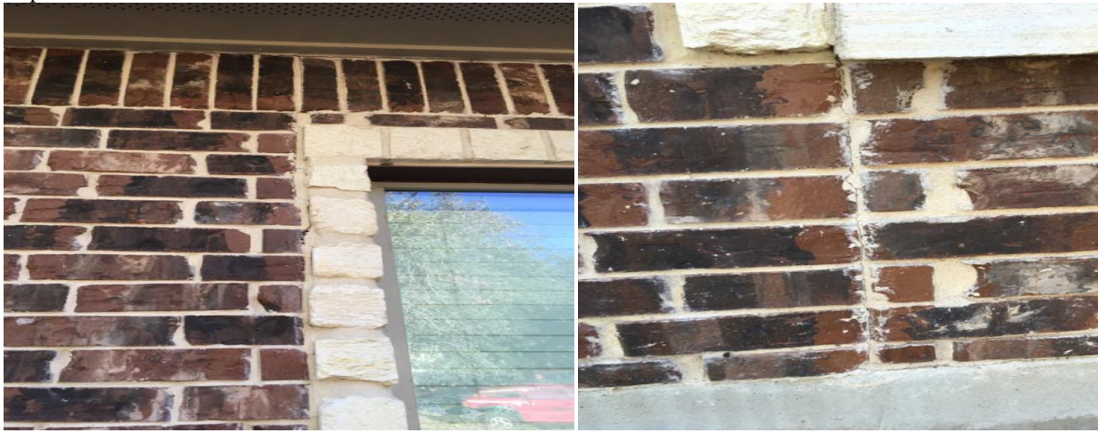
Expansion Joint With Lose Mortar
