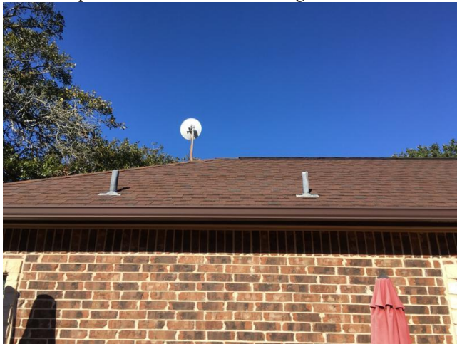
Rusted exposed nail heads need roofing cement.
